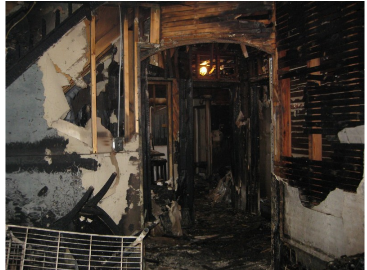
Photo of Rachel's hallway after the fire
